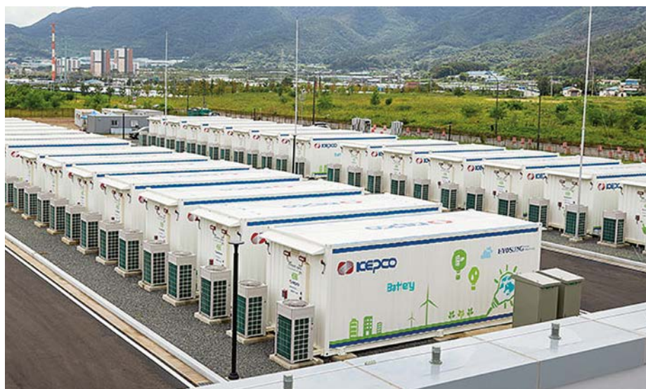
A 978 MW battery energy storage system in Korea belonging to Korea Electric Power Corp.
